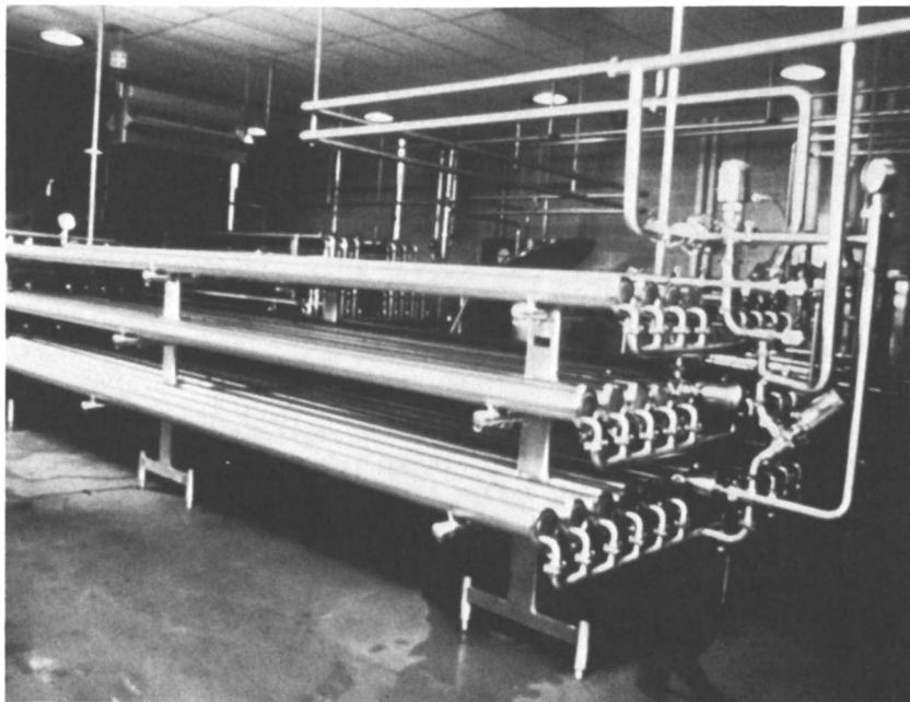
Figure 3. Production scale sanitary RO/UF system.
